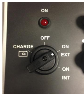
f-POD ON EXTERNAL BATTERY
