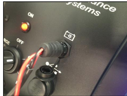
BATTERY CHARGER CONNECTED
